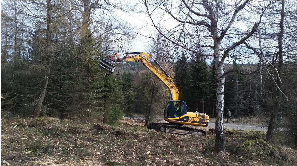
Fig. 1: Example of site preparation for conversion of substitute blue spruce stands. Standing whole trees are processed by chipper and therefore biomass is equally distributed on area for planting of target species.
