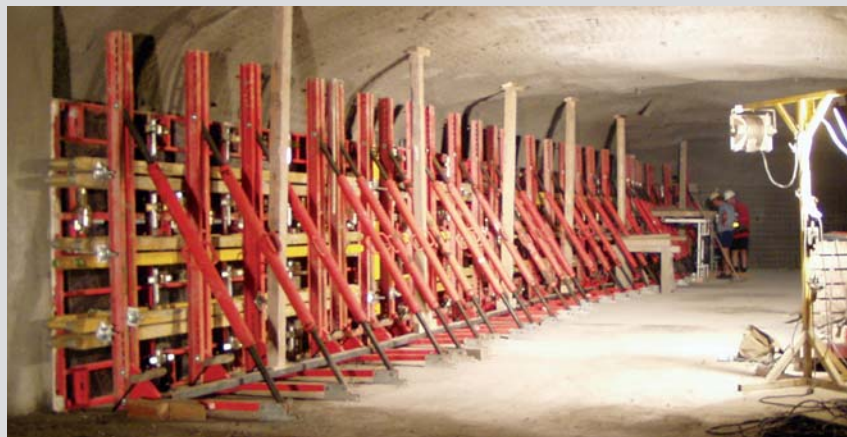
The "Realisation of Closure of Chambers at the Richard Repository" project; the construction of the inner wall of the hydraulic cage.
